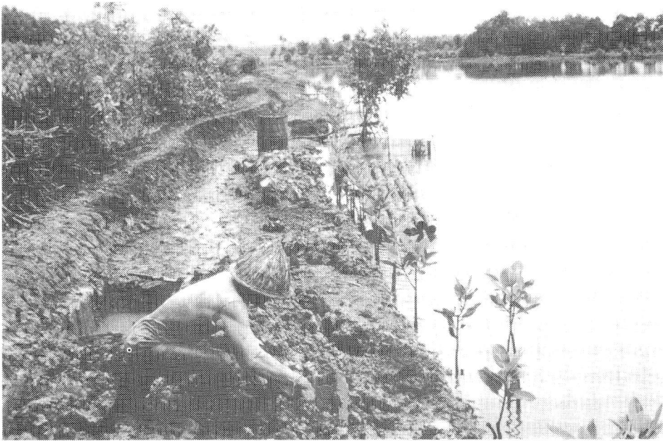
Fig. 1. A fishpond and pond repairing. Note the plantation of mangrove seeds at the water edge. Madura. June, 1981.
