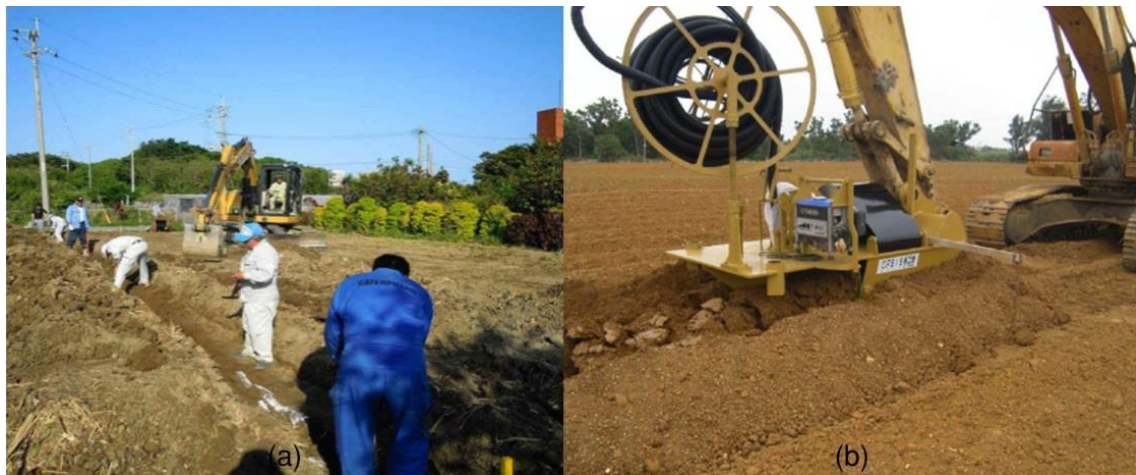
Figure 2.9. Installation of OPSIS lines a) Manually laying out lines, b) Use of a machine to layout the lines
