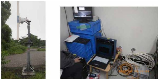
Fig.7. Kurokami antenna unit (left), control monitoring unit (right)
