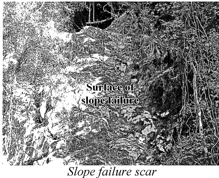
Fig. 4 Pattern diagrams and state of erosion and slope failure observed at sample point No.25.
