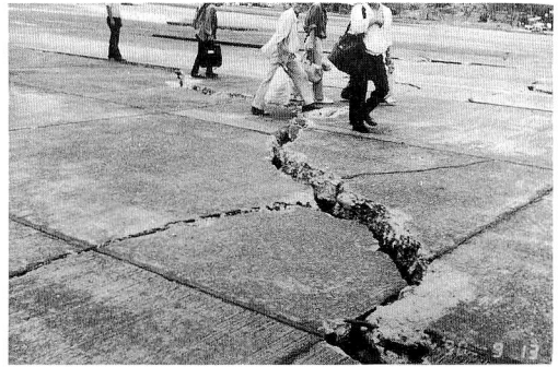
Photo 29 (b) Crack in runway of air port
