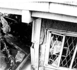
Photo 28 (c) Inclined Wooden House
