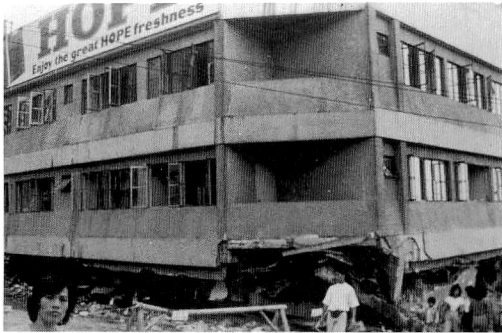
Photo 21 (a) ROYAL INN First story columns were collapsed.
