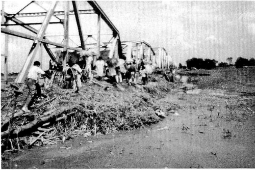
Photo 2 (a) Falldown bridge on the way from MANILA to DAGUPAN
