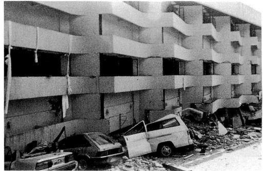
Photo 16 (b) HOTEL NEVADA after the earthquake
