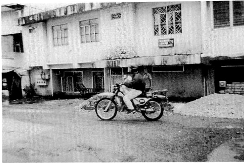
Photo 11 Subsidence of residential house
