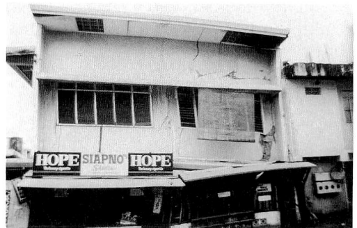
Photo 8 (a) Inclined wooden house
