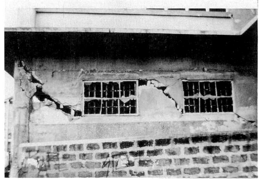
Photo 24 Little Angeles Nursery School near FRB HOTEL (Shear cracks of Bamboo and clay wall)
