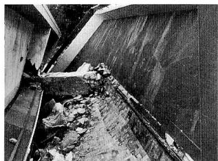
Photo 18 (g) HYATT TERRACES HOTEL Lain down column
