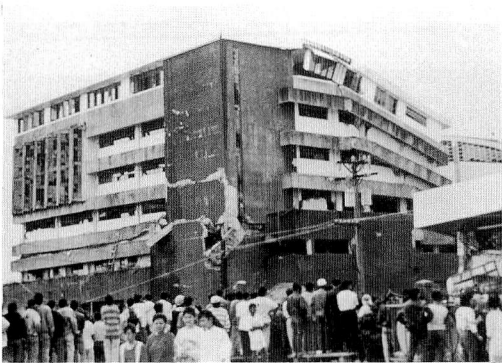
Photo 23 (a) University of BAGUIO College of Commerce (south and east view) Fifth story columns were collapsed
