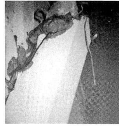
Photo 23 (c) University of BAGUIO College of Commerce Column failed due to shear
