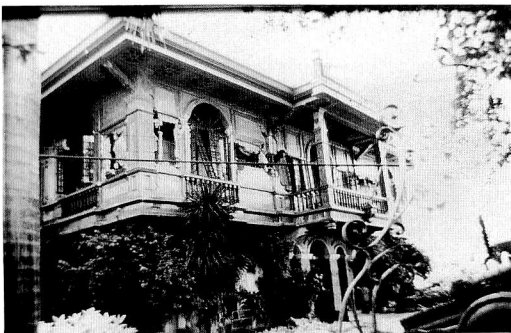
Photo 3 Residential house on the way to Dagupan The earthquake caused much damage so that the house is not able to use.
