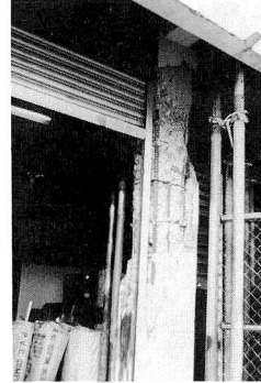
Photo 26 (b) BAGUIO CITY EXPORT PROCES- SING ZONE (Factory No.1) Concrete cover of some columns fell down.
