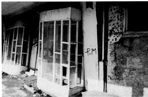
Photo 12 (a) Subsidence of shopping house
