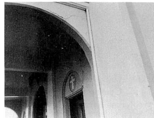
Photo 25 (b) BAGUIO CATHEDRAL (Entranse) Many small cracks were observed.
