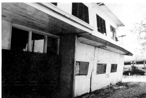
Photo 8 (c) Inclined wooden house
