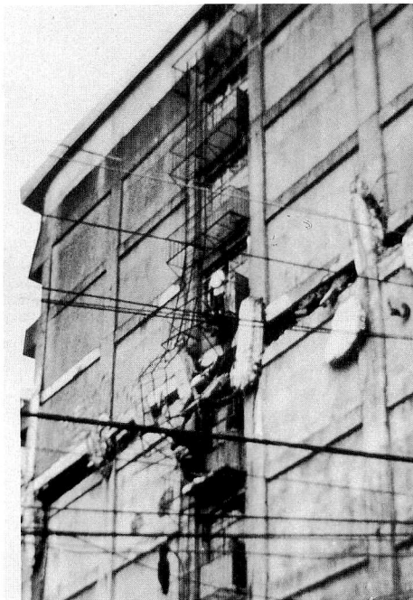
Photo 23 (b) University of BAGUIO College of Commerce (West side view) Fifth story columns have no framed wall.
