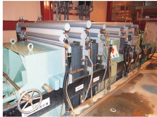
Fig. 1. Water desalination plant on Yoronjima Is.
