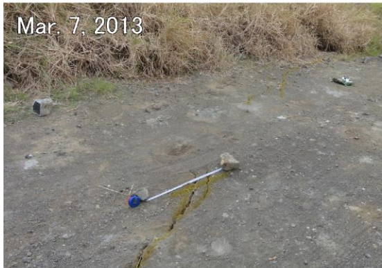
f. Open cracks on the nearby road (taken by T. Tanada).
